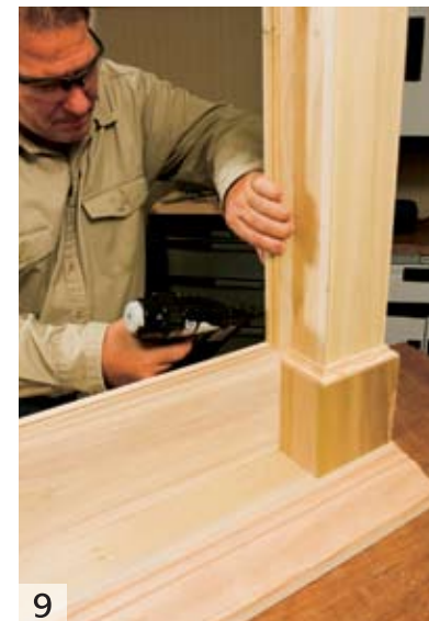
The inside trim molding conceals the outside edge of the tile border. Miter the inside corners of this molding and attach it to the inside edge of the backer boards with 1-1/4-in. brad nails.
