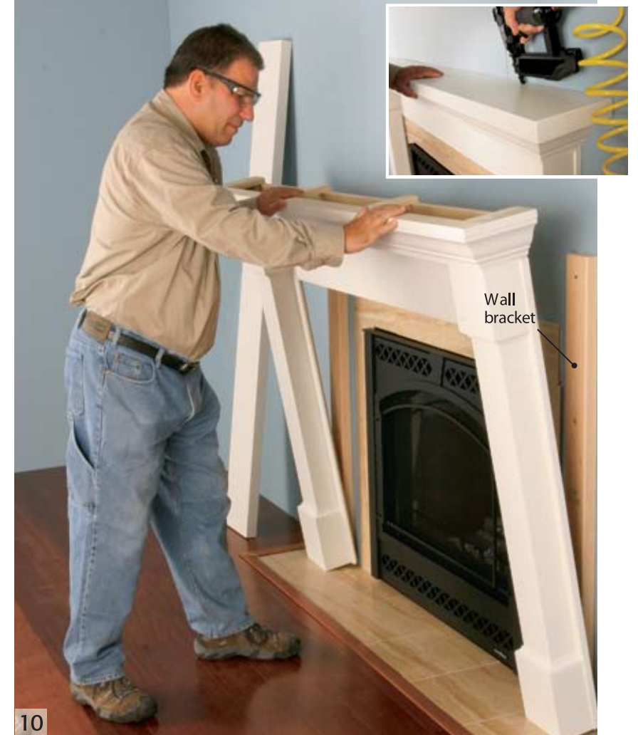
Mark the outside edges of the posts on the wall, measure in 1-3/4 in. from those marks and attach the wall brackets to the wall. Then slide the mantel over the brackets and attach it with 2-in. brad nails. Next, attach the middle of the mantel back to the wall. Finally, attach the top with 2-in. brads (inset).
